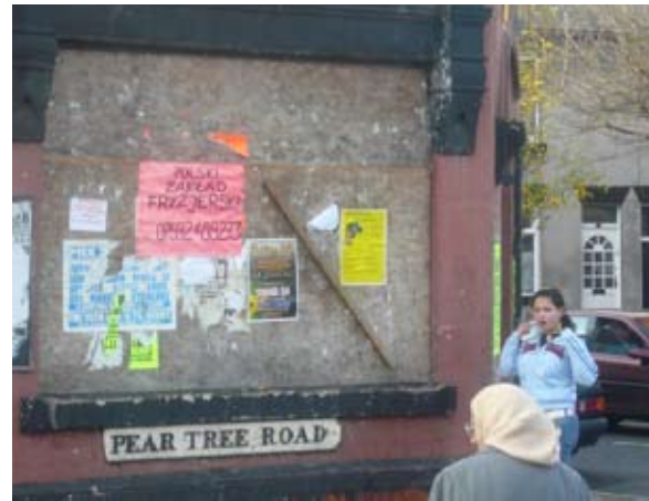
The derelict Normanton Hotel at the heart of Normanton
